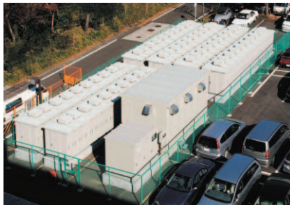
Electric power storage system utilizing lead storage batteries in the Research Division
