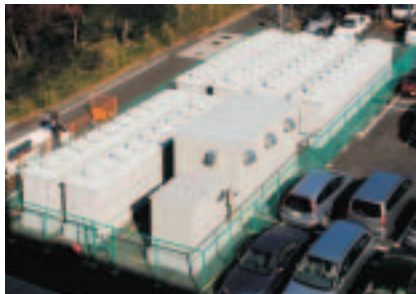
Electric power storage system utilizing lead storage batteries in the Research Division
